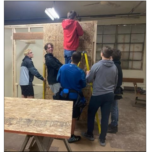
walls up to use for electrical & plumbing lessons.
