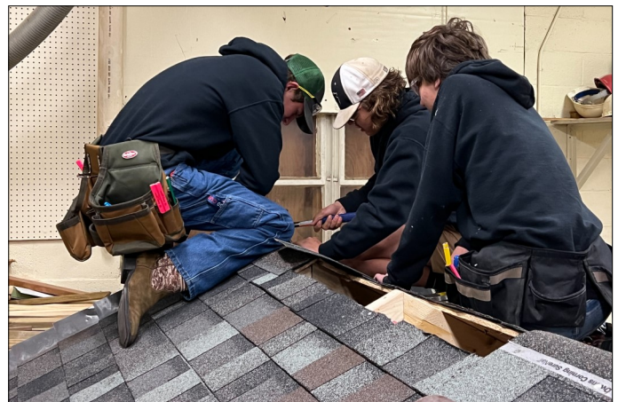
With generous donations from ABC Supply in Freeport, CareerTEC construction trades students learned how to shingle a roof in the fall.
